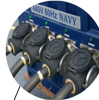
Onshore Power Supply
