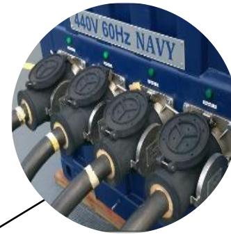
Onshore Power Supply (MR1)
